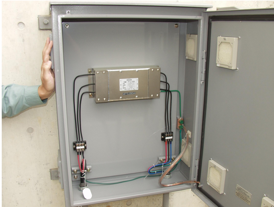
Figure 49 Improper Filter Configuration
