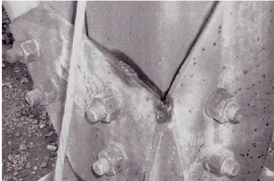
Figure 13 Weld on Galvanized Metal of a Receiving Antenna Tower
