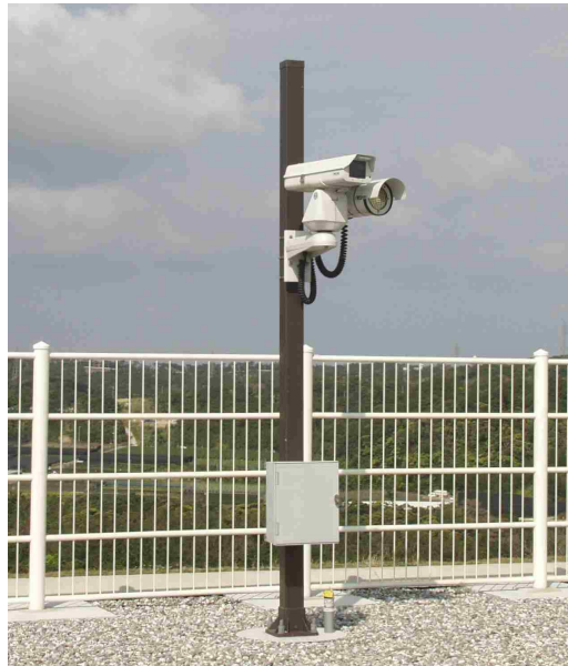
Figure 55 Security Camera Powered by a Noisy Switching Power Supply
