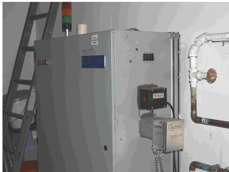
Figure 45 Filter Installation to Suppress Motor-Controller Noise
