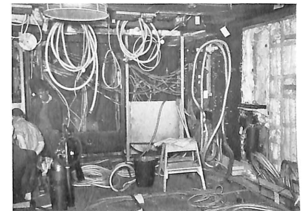
FIGURE 5—Cable runs in CIC, U.S.S. ANTIETAM.
